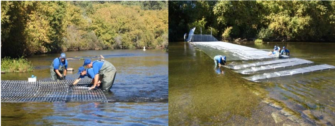
Figure 10. Inserting a connecting picket between two adjoining panels (left); continuing across the river channel (right).
