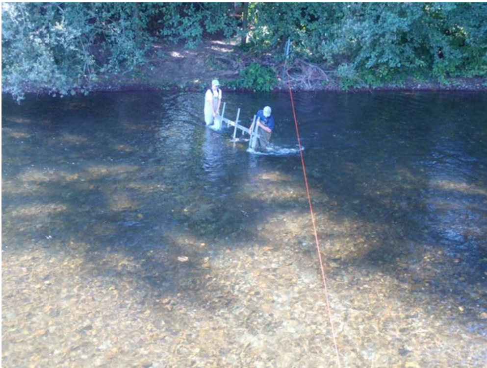
Figure 5. Use of a reference line, such as a cable or string, stretched across the river to guide substrate rail installation.
