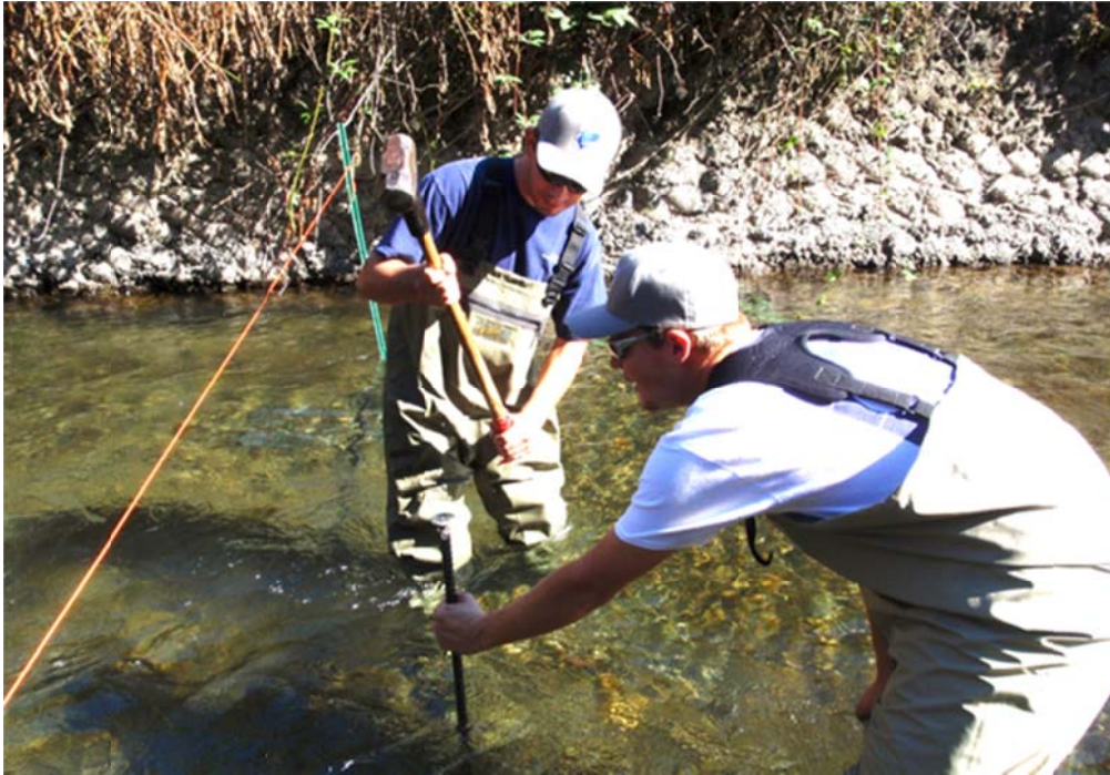
Figure 6. To secure each rail section to the river bottom, drive the rebar pins through the holes on the ends of each leg along a substrate rail section.
