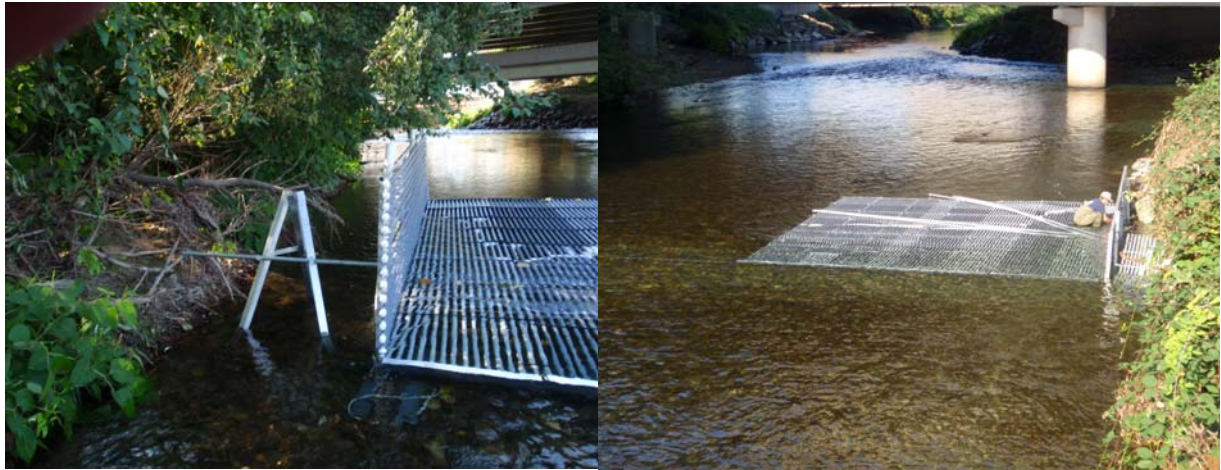
Figure 8. Installed A-frame, associated rigid weir panel, bulkhead and first resistance board panels.
