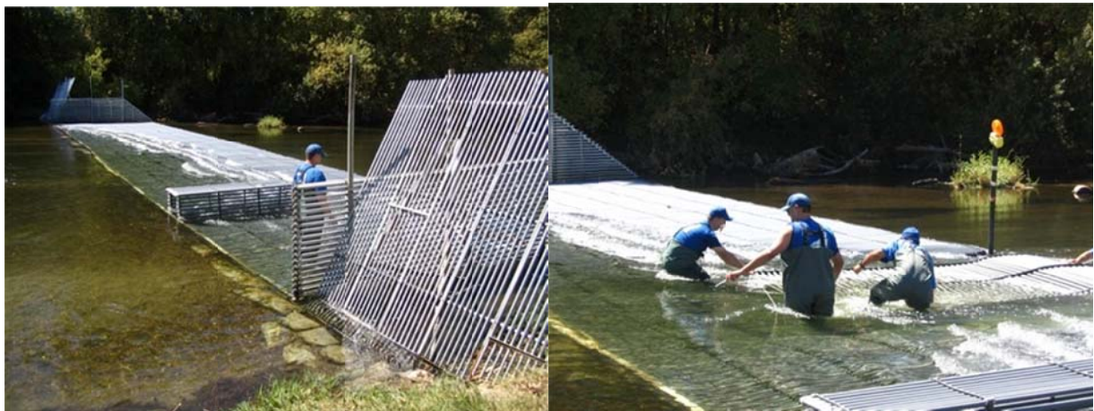
Figure 11. Completed weir installation (minus live trap)(left); installation of the boat passage cap panel (right).
