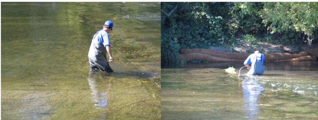
Figure 4. Clearing excess sand and gravel deposited on top of the substrate rail during high flow (spring) conditions (left); and attaching the substrate rail cable (right).
