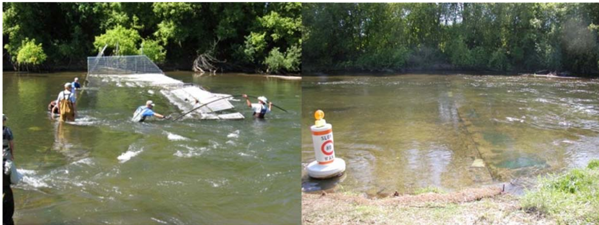
Figure 46. Technicians removing connecting pickets and unhooking a resistance board panel (left); and a weir site after removal with the substrate rail left in place (right).
